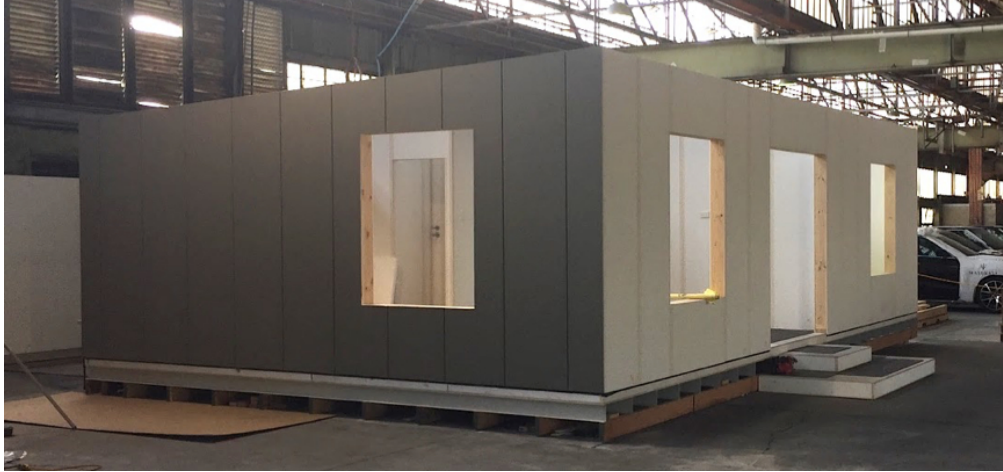
Figure 1. Prototyping of SIP walling system for the LP13 project 145x68mm (150 x 150 DPI)
