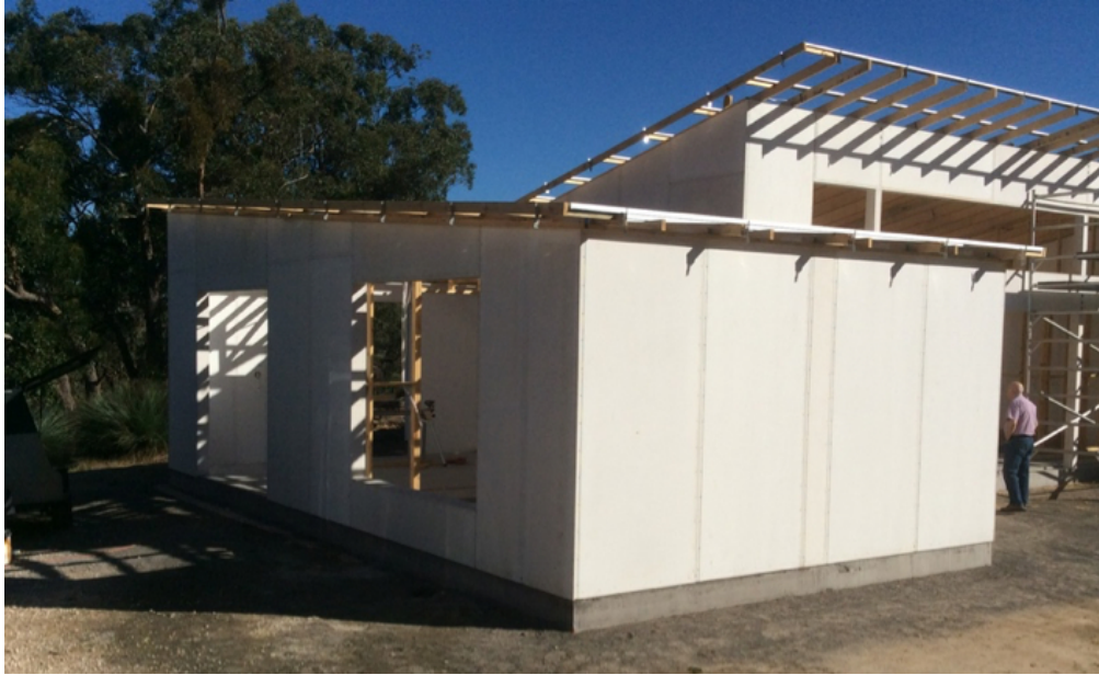
Figure 7. House in Adelaide Hills under construction with industry partner’s SIP wall system
