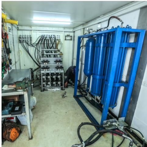
Figure 3: The installed hydraulic circuit in Gaza
