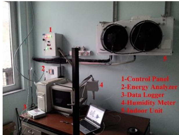
Figure 2: Indoor unit of the heat pump
