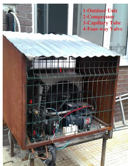
Figure 1: Outdoor unit of the heat pump
