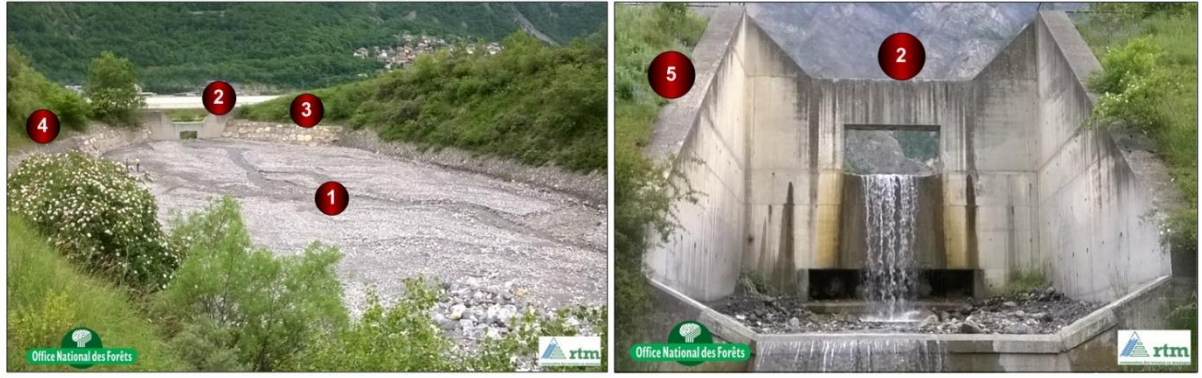
Figure 1. Claret retention system: (1) retention basin, (2) retention dam, (3) lateral dykes, (4) access track and (5) downstream counter dam. Upstream view (left panel) and downstream view (right panel) © ONF-RTM/S. Carladou May, 23 rd 2018.
