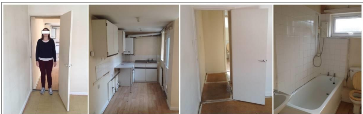
Figure 3.3 – Images showing problem areas: (far-left) ground floor access way; (mid-left) ground floor kitchen; (mid-right) first floor access way; and, (far-right) first floor bathroom
