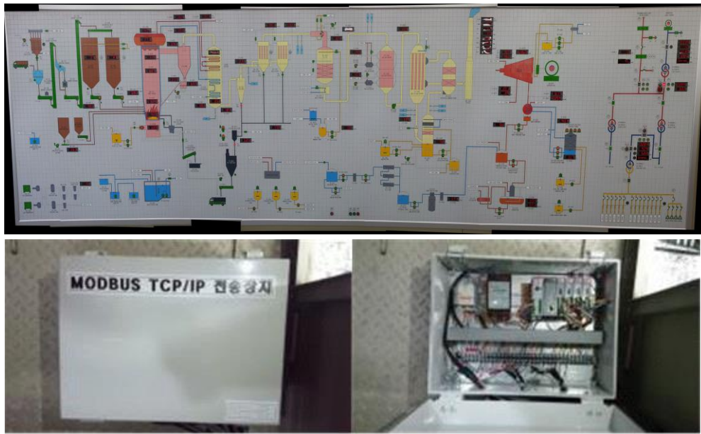
Figure 3. Mosaic panel of coal-fired power plant and signal bypassing device
