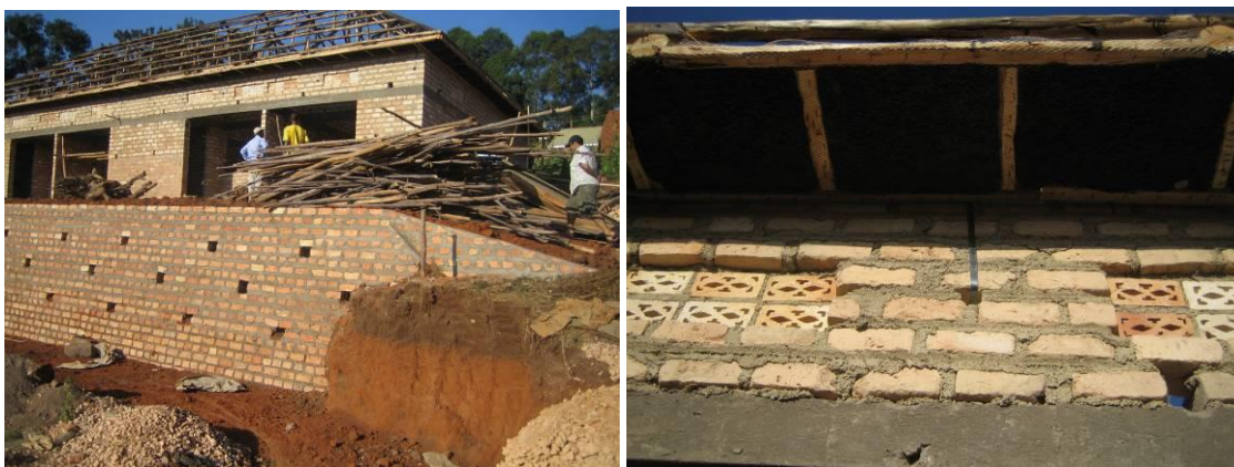
Figure 5: Mortar thicknesses of up to 30mm is normal for brick walling (Uganda)
