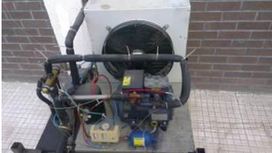
Figure 2. Outdoor unit of air to air heat pump
