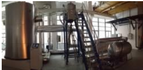
Fig.4 Photograph of the thermal storage tank
