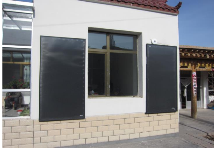
Fig. 2: Solar air heaters on the south wall
