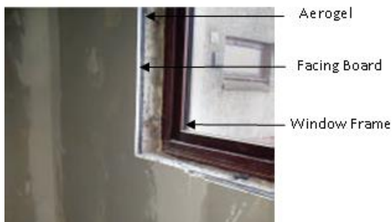
Figure 48: Spaceloft® aerogel used for building wall insulation (AA, 2011a)
