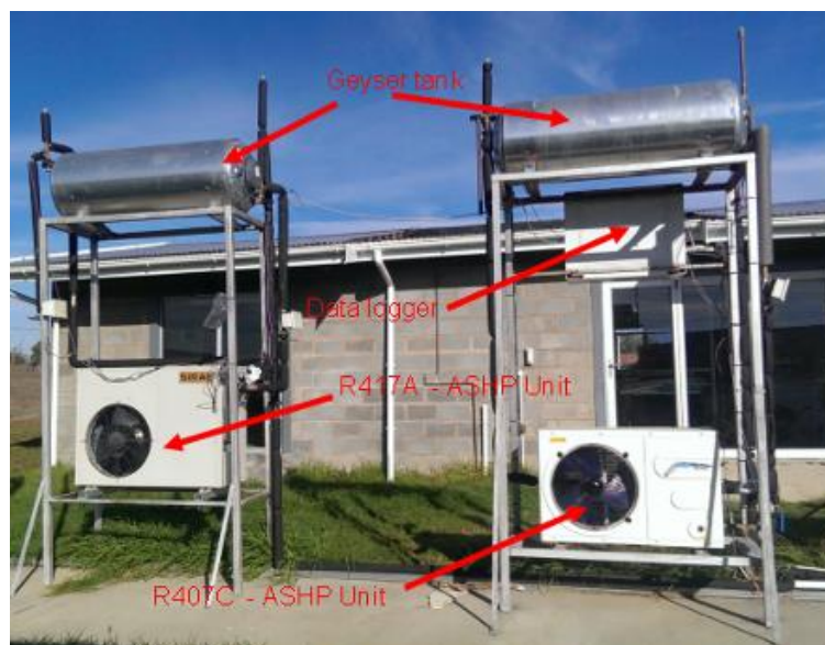
Figure 6: Illustrates the ASHP water heater and data logger installation setup
