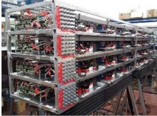
Fig. 5: The final converter structure with the four series connected NPC pairs stacked on top of each other.
