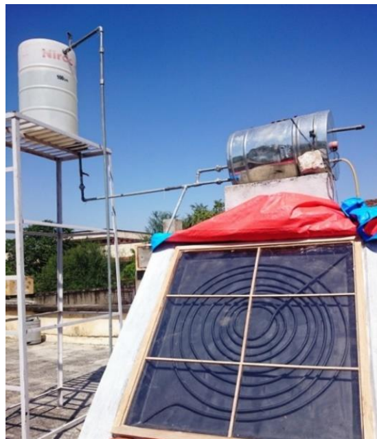
Figure 1: The building integrated solar water heater (BISWH)
