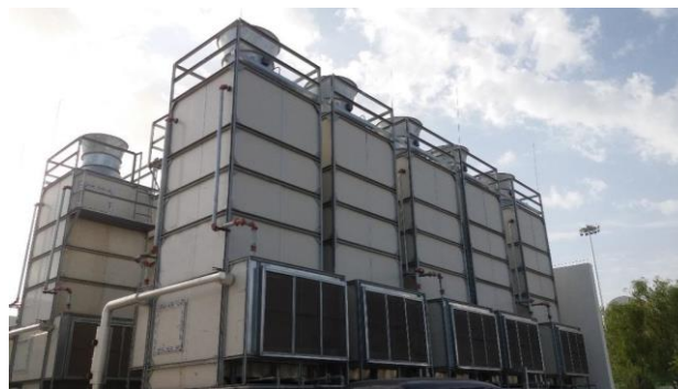
Figure 1: High-temperature evaporative water chiller at refrigeration station of Dunhuang Airport
