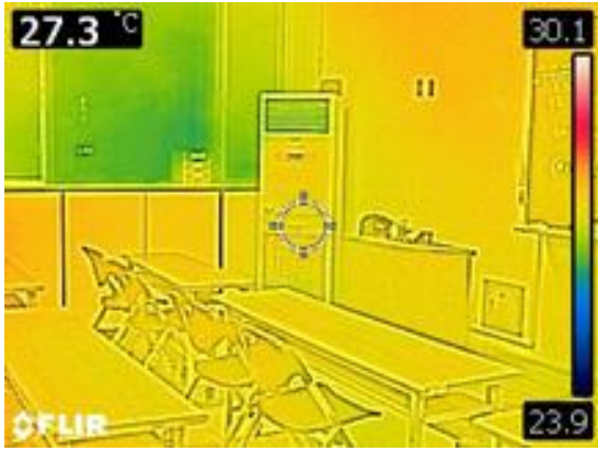
Figure 5a: Windows in the classrooms dissipate heat at night
