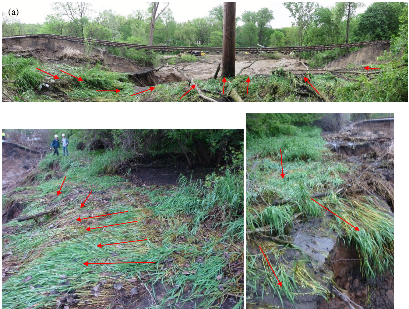
Figure 13. View of the failure and the reeds uphill of the embankment. The arrows are parallel to the direction of the fallen reeds that bent and broke during the abrupt emptying of the ponding water and fell on the ground with their orientation pointing to the initiation point of failure. (Fig. 13a by Karl Jansen, ceephotos.com)
