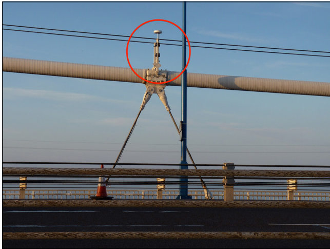
Figure 9. A GNSS antenna located on a Severn Bridge suspension cable
