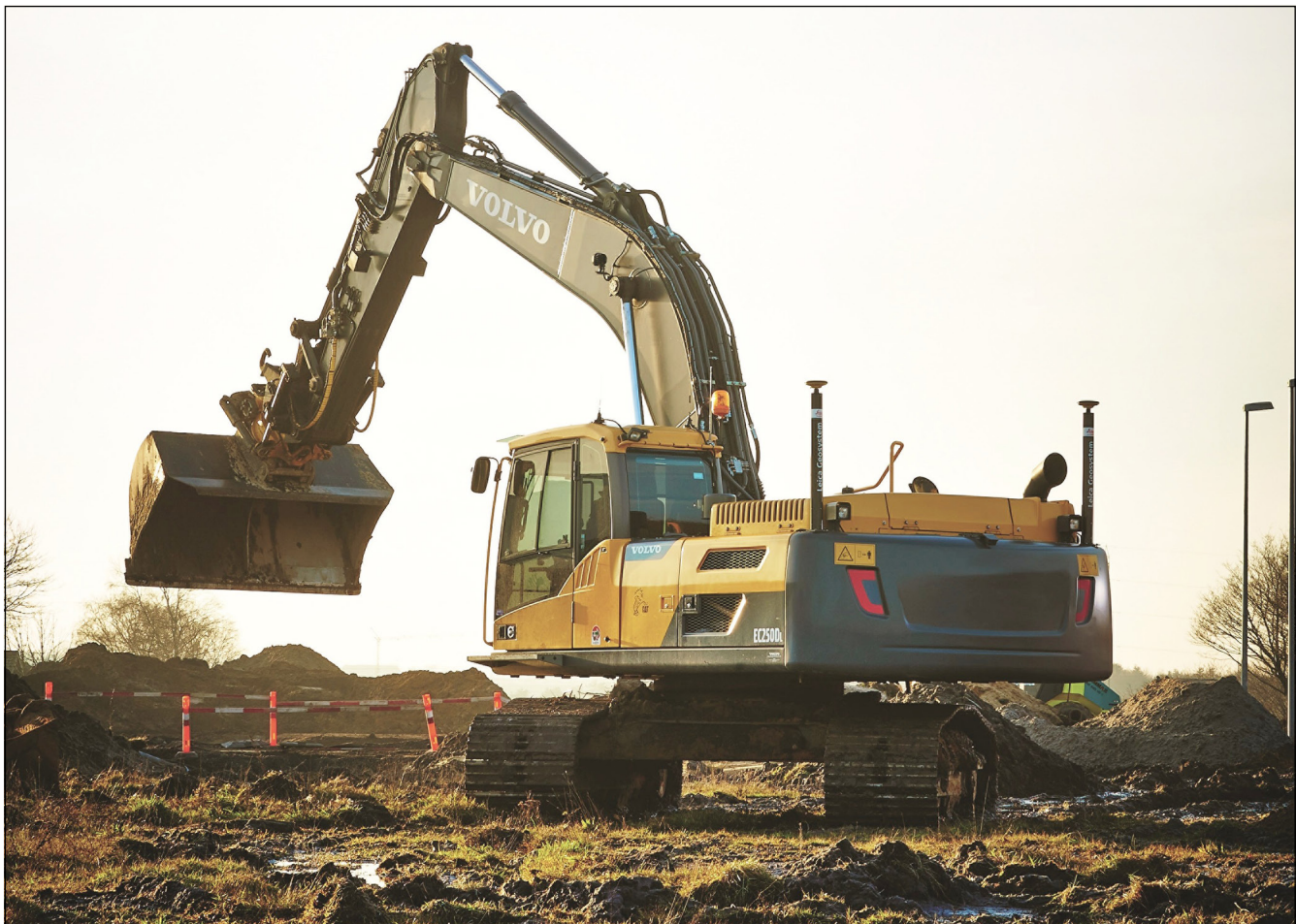
Figure 8. An excavator using RTK GNSS for control – notice the lack of setting-out sight rails and batter rails (courtesy Leica Geosystems)
