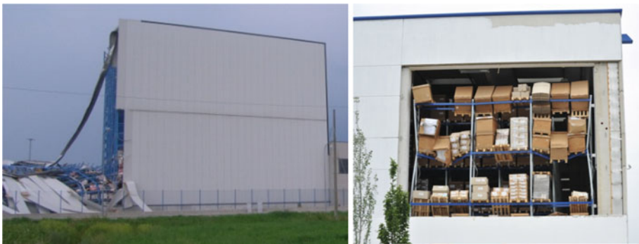
Fig. 19 Collapse and local failures attributed to the failure of rack systems
