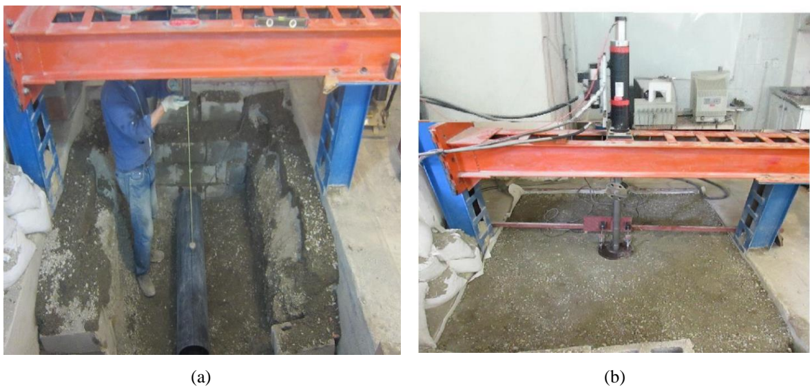
Fig. 7. Photograph of (a) pipe installation in trench (b) test installation prior to loading include reaction beam, load plate, hydraulic jack, load cell and LVDTs
