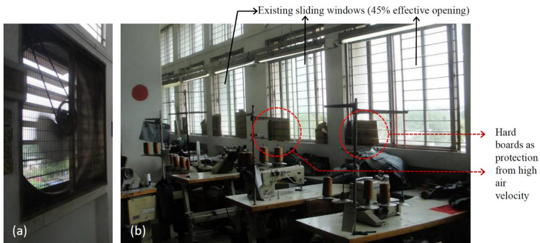
Figure 3. (a) Extract fans at ventilation outlets (b) Sliding windows at ventilation inlets with hardboard to protect workers from direct air flow
