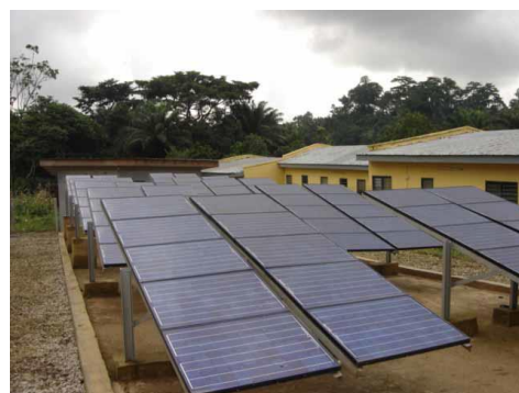
Figure 4: Solar PV at Ilaje, Ondo State of Nigeria
