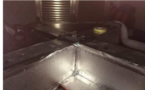
Figure 4: Flow ducts in the indoor room
