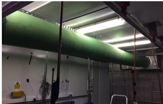
Figure 2: Experimental test facility with air distribution via fabric duct.
