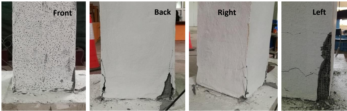
Fig. 14: Damage state at the end of the test for SRG3.
