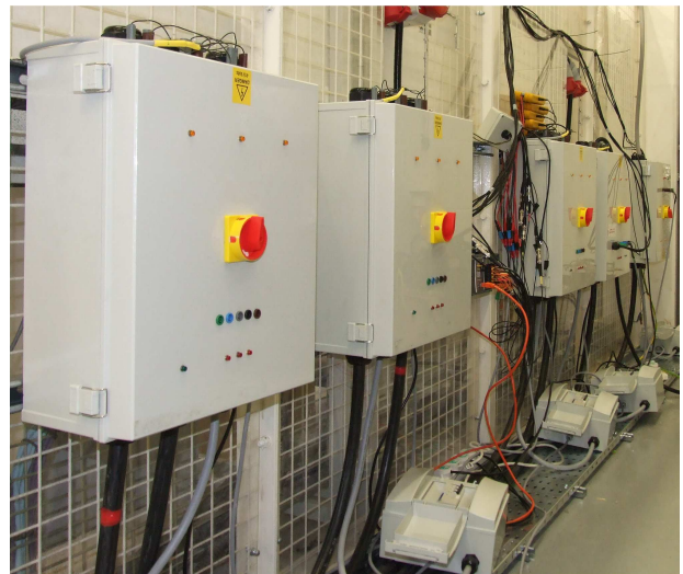
Fig. 1: Photograph of the experimental facility.
