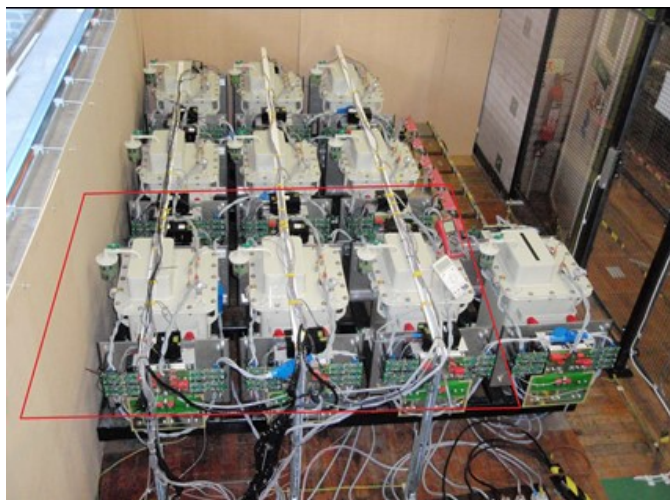
Fig. 9. UNIFLEX-PM power converter in place for low voltage testing: (a) complete 12-cell setup for 3-phase 3-port operation, (b) highlighted cells used for single-phase 2-port operation.
