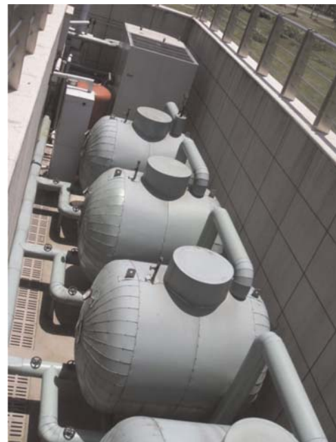
Figure 5. Hot water storage tanks.
