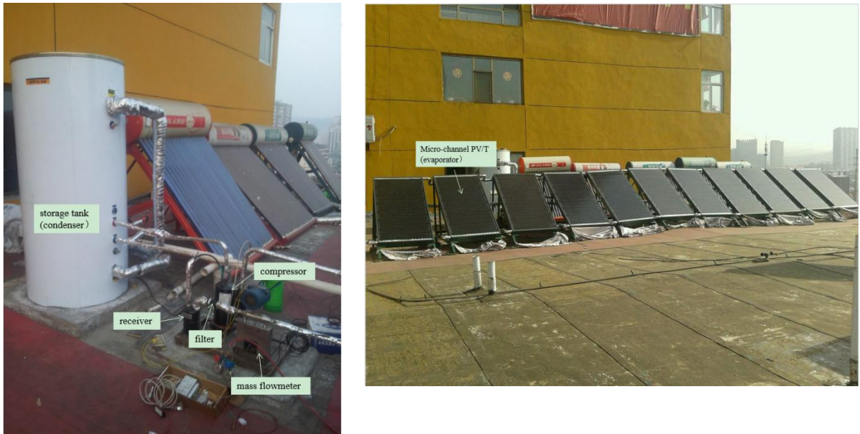
Figure 2: PV/micro-channel-evaporator modules based heat pump system set up
