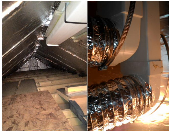
Figure 4: The novel heat recovery system fixed beneath the roof and flexible ducts.
