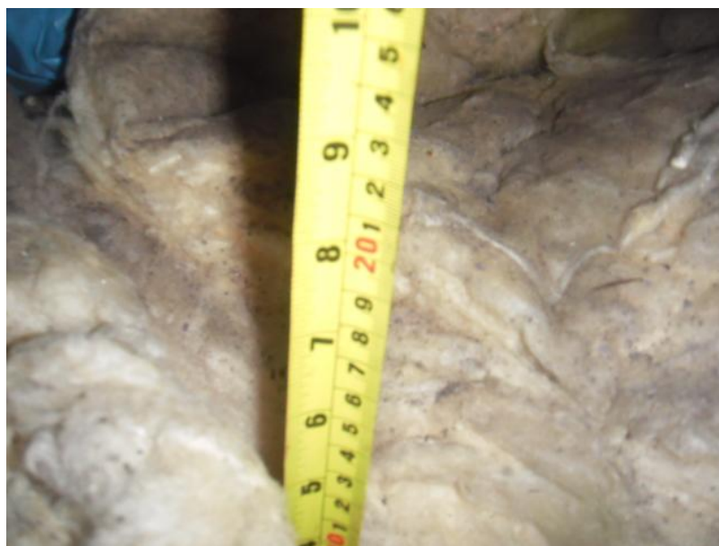
Figure 1: 100mm glass wool insulation in the loft space of the residential building.
