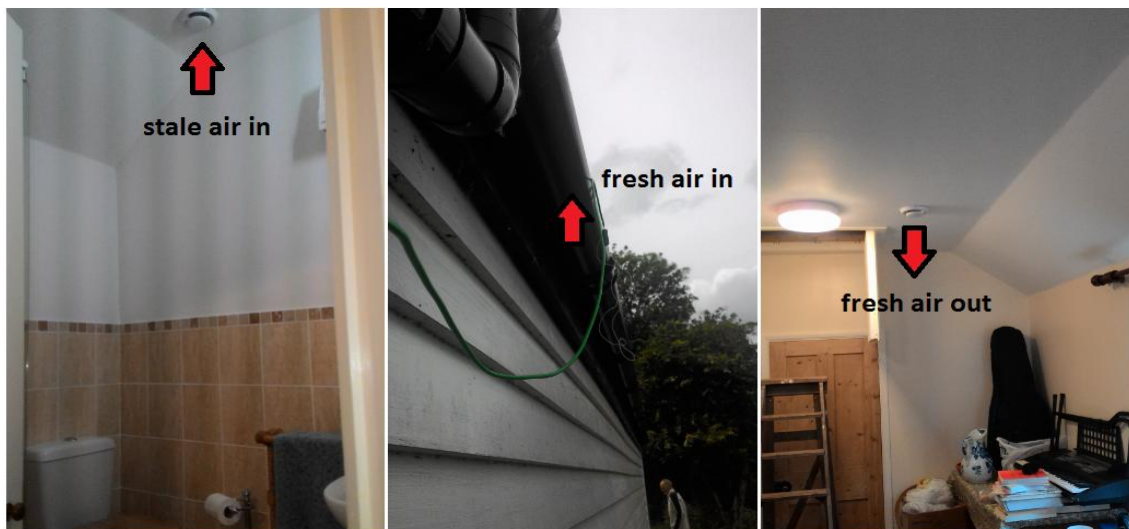
Figure 5: Inlet and outlet ventilation ducts in the test house.
