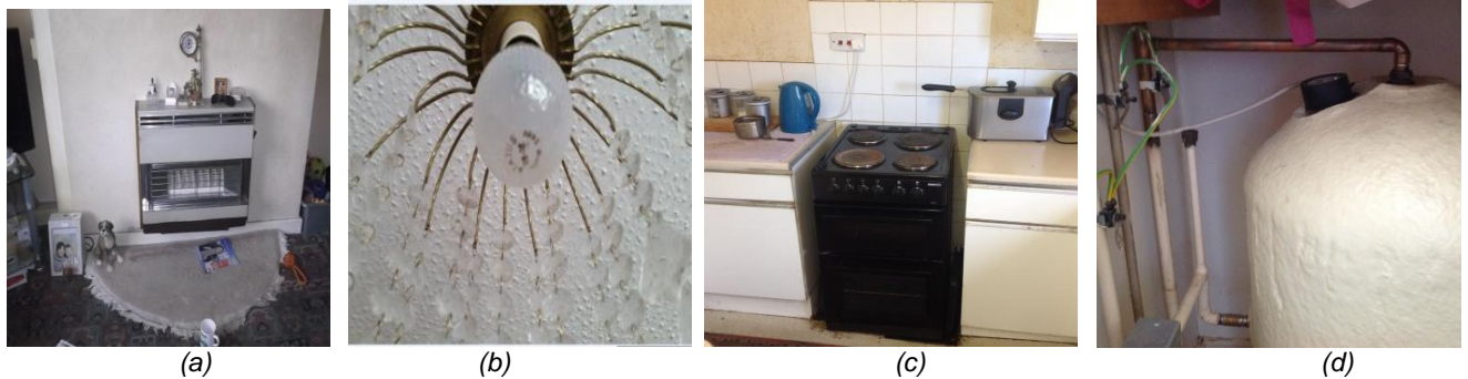
Figure 6: (a) Electrical central heater, (b) Incandescent light (100W), (c) electric cooker, (d) No insulated pipes
