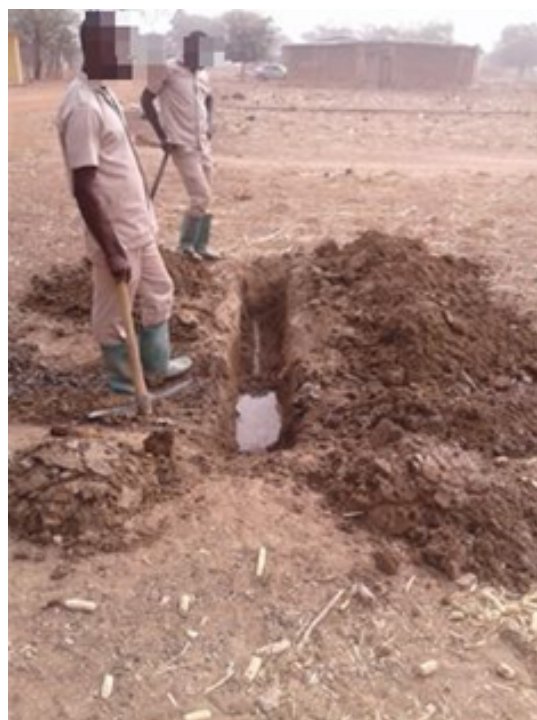
Source: Field survey, February 2018 Fig. 10. Staff of GWCL, repairing a leaking pipe in Navrongo, Kassena Nankana Municipality
