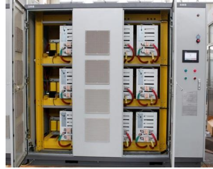
(b) Nine-level high voltage inverter
