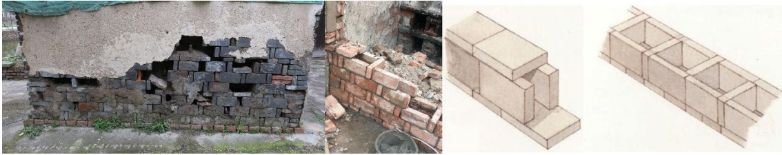
Figure 5: rowlock wall in Feng Xian is the local choice for residential buildings even today.
