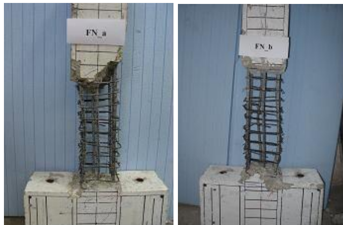
Figure 7 Specimens FN_a and FN_b after removal of damaged and fragmented concrete
