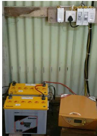
Figure 6: Project setup: Inverter, Batteries, Smart Switches and MCBs
