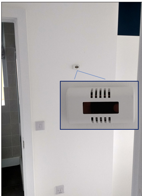
Figure 1: An EnOcean temperature and relative humidity sensor installed in one of the properties. A magnified view is shown in the inset image.
