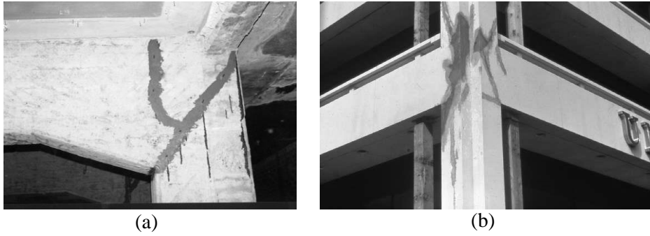
Fig. 1 Application of the (a) epoxy resin and (b) cement grout injection in beam-column joints
