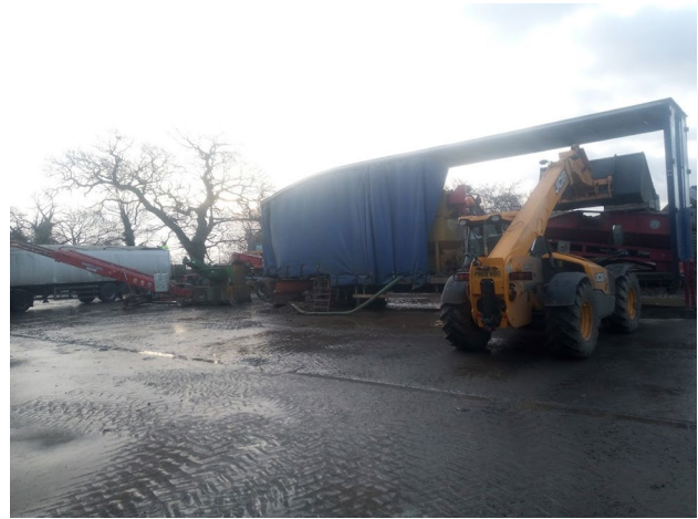
Fig. 8 Farmer invention: Mobile potato washer. Farmer description: “This is the biggest of our recent projects, a mobile potato washer. Most washers need a hopper and elevator to feed them, and so are static. We built one into a 45' curtain-sided step frame trailer. A second-hand donor grader provided a sensor-controlled hopper and coils and all of the cross conveyors. This is fed directly with the forklift, the coils remove any loose soil, then they go up a flighted elevator surplus from a redundant box filler on farm, into a 3×1 m barrel washer sourced from a redundant packhouse in Ireland. On exit they are rinsed onto a picking table and head out through the headboard of the trailer into another flighted elevator which feeds them into a remote-controlled telescopic elevator and into the lorry. The green section in the line is a destoner, which we put in the line for various customers, but not all. The pickers are protected from wind, rain and cold, and now have much more comfortable working conditions... Cost £42,000. Saving minimum £25,000/year.”
