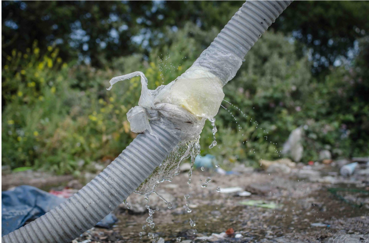
Figure 4: A leaking drinking water pipe in the Calais camp, presenting a risk of supply contamination. One water tap tested positive for pathogenic bacteria indicative of faecal matter.
